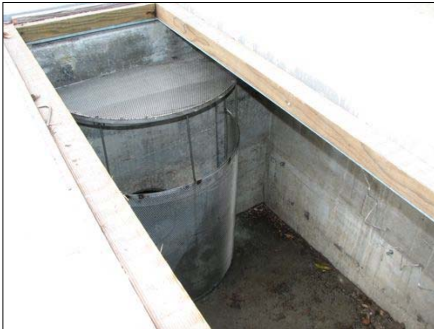
Figure 1: CPS inside catch basin
